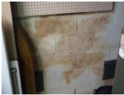
11 view of moisture penetration under chimney
