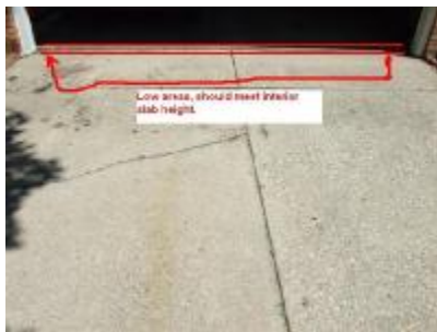
8 Garage door no positive seal
