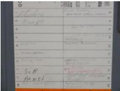
3 Partially unlabeled electrical panel roster
